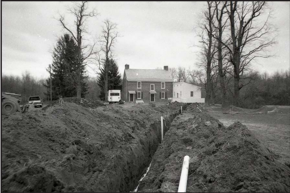
Photograph 3.14. Electrical and sewer line trench (F). View looking north from parking lot area towards the house. (Photographer: Vivian Braubitz, 2000) [Hunter Research Inc. Neg.00015/1:20]
